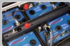
Maintenance free Batteries
